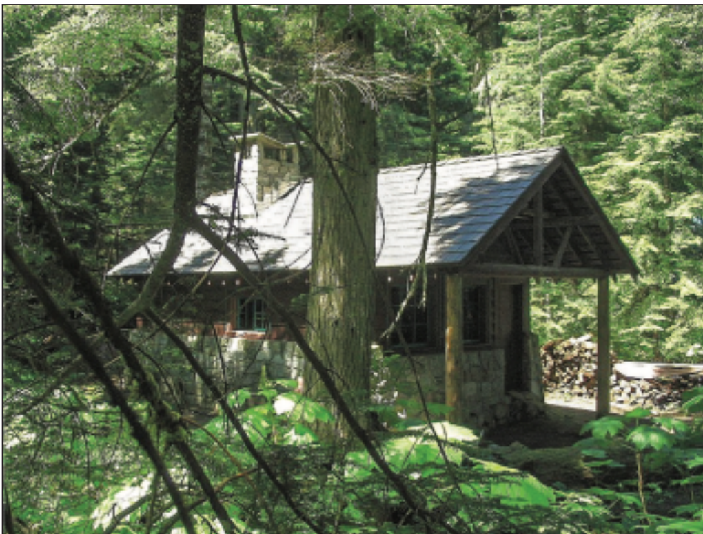
Figure 8—A tree fell during a storm and destroyed most of the original roof of this 1950 recreation residence at the Denny Creek tract of the Mt. Baker-Snoqualmie National Forest in the Pacific Northwest Region. The new roof structure and materials match the appearance of the historic roof, although the structure was strengthened to meet code requirements for snow loading.
