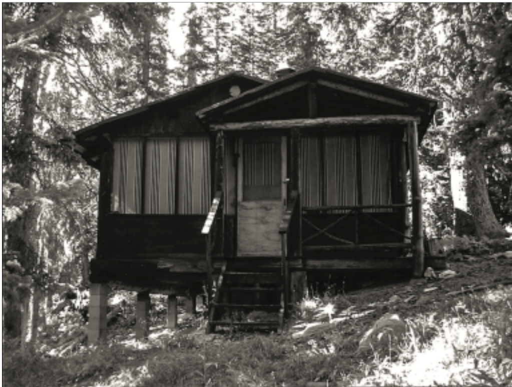
Figure 24—This recreation residence at the Cascades tract of the Medicine Bow National Forest in the Rocky Mountain Region was built in 1927 on a concrete block post and beam foundation—a relatively inexpensive method to support a building on a sloping lot. This foundation may not meet current building codes.
